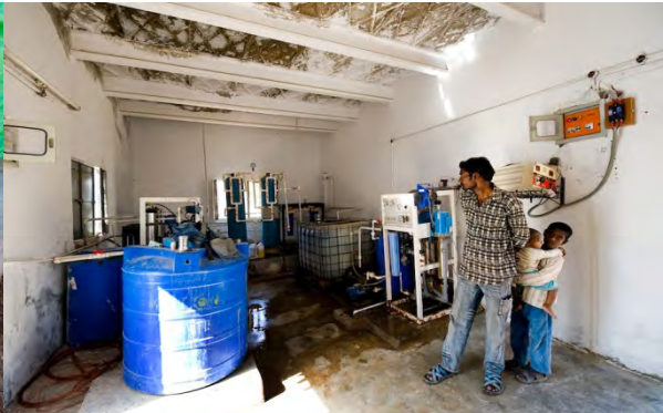
Picture 19: Water purification/filter plant
