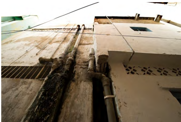
Picture 18: Poor condition of sewerage pipes
